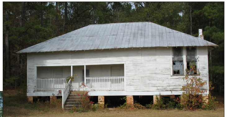
South exterior structural restoration. Small photo to the right shows this structure before restoration. Large photo below shows the restoration in progress.
